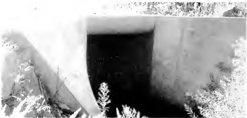
FIG. 22. Warped wing headwall with rounded-lip crown at entrance to concrete box culvert
